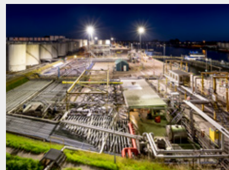
Tank storage Standic B.V. | Dordrecht | Netherlands
